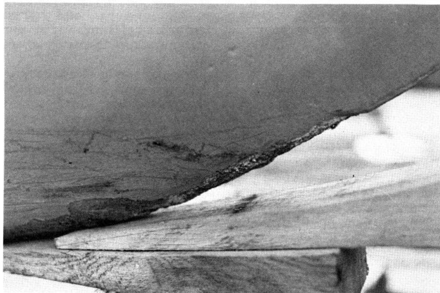
Minor gouges in the fiberglass shell surrounding an encapsulated keel should be repaired to prevent long-term problems
